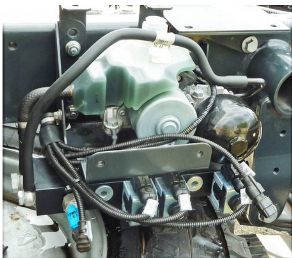
APU, Diff Lock Hydraulic Pump
