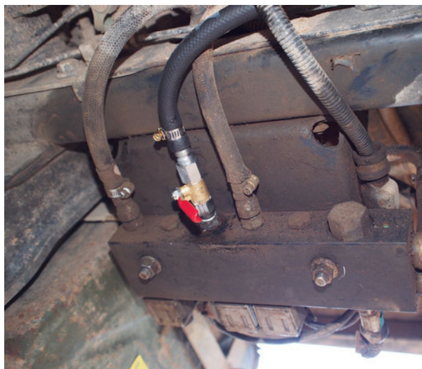
Tap added to CDL line to "fix" leak into transfer case
