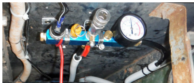
onboard air manifold
